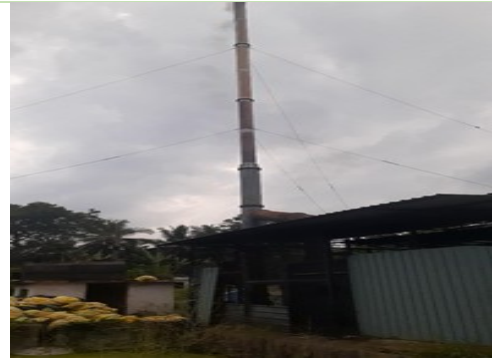
Incinerator for infectious waste management
